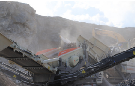
Multi-use for primary scalping and screening.
