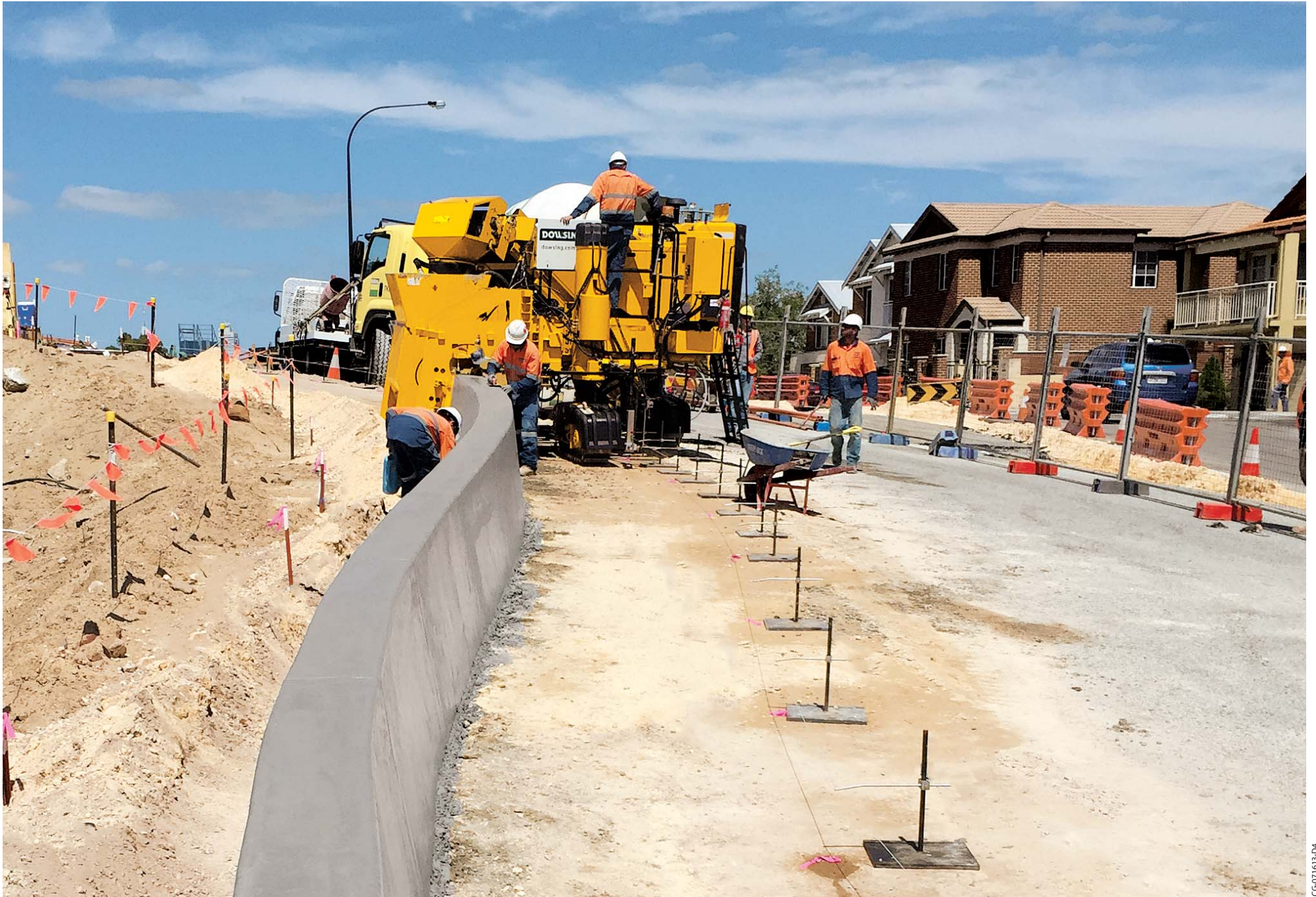
A GT-3600 slipforms variable ranging in height between 34.8 to 50 inches (885 to 1270 mm) on a project in Perth, Australia.
