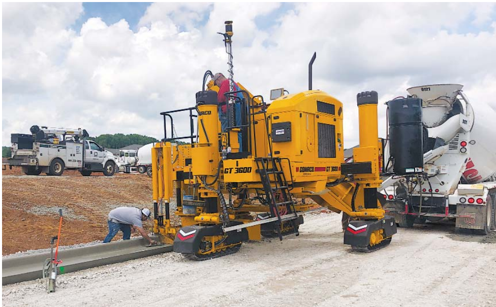
A GOMACO Xtreme GT-3600 slipforms curb and gutter for a new subdivision using 3D machine guidance.
