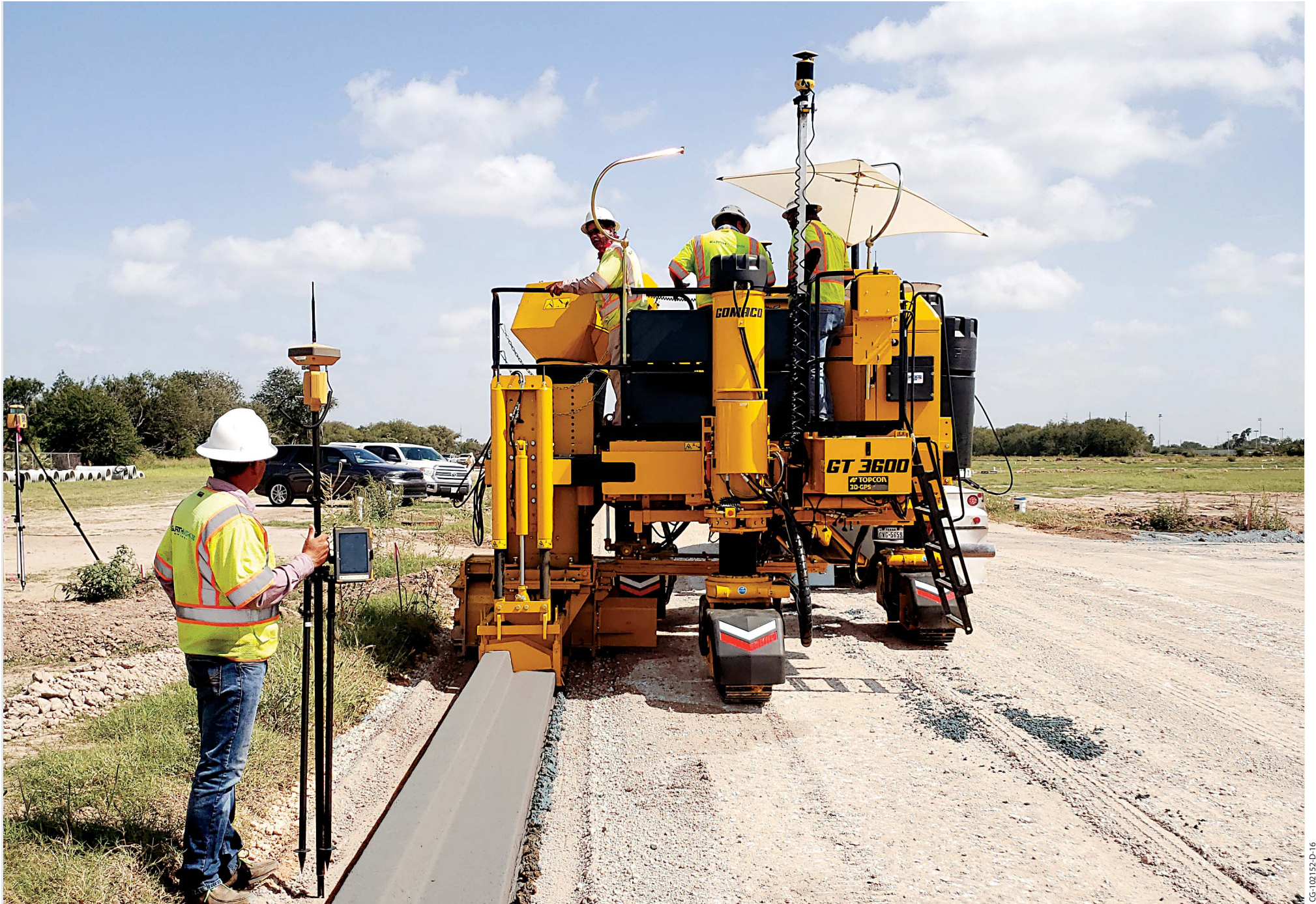
An 18 inch (457 mm) curb and gutter is slipformed using 3D machine guidance by the Xtreme GT-3600 in a new residential development.
