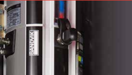
Sandvik central greasing unit
