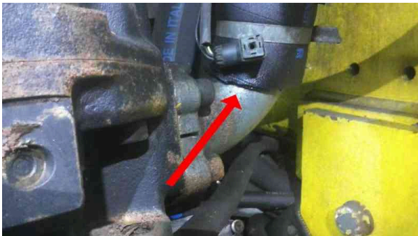
suction hoses are leaking
