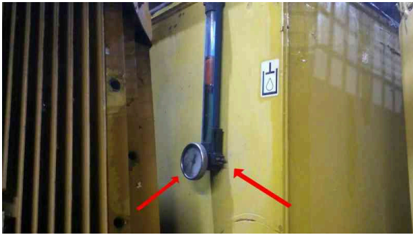
Oil level sensor and temperature gauge not working, have to be replaced
