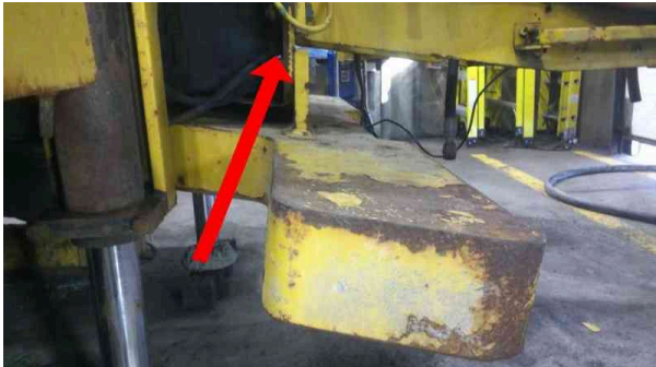
Rear counter weight bracket crowked,need to be repair
