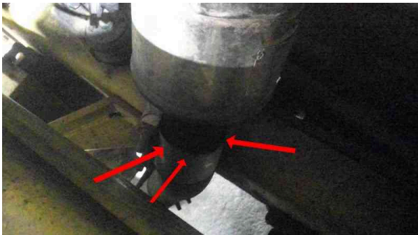
Exhaust clam smoke a lot and need to be replace
