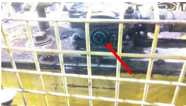
Filters gauge broken, need to be replaced
