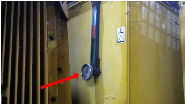
Gauge not working, have to be replace
