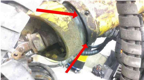
Very loose more than 1/4 inch, need to be replace
