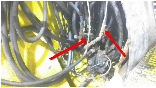
Cut wires under the operator console
