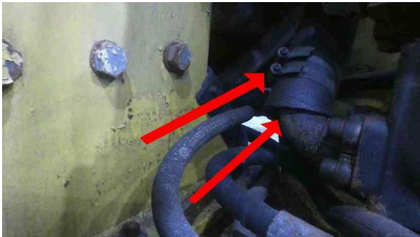
Succion hoses are leakings and need to be replace,wrong clams,wrong hoses
